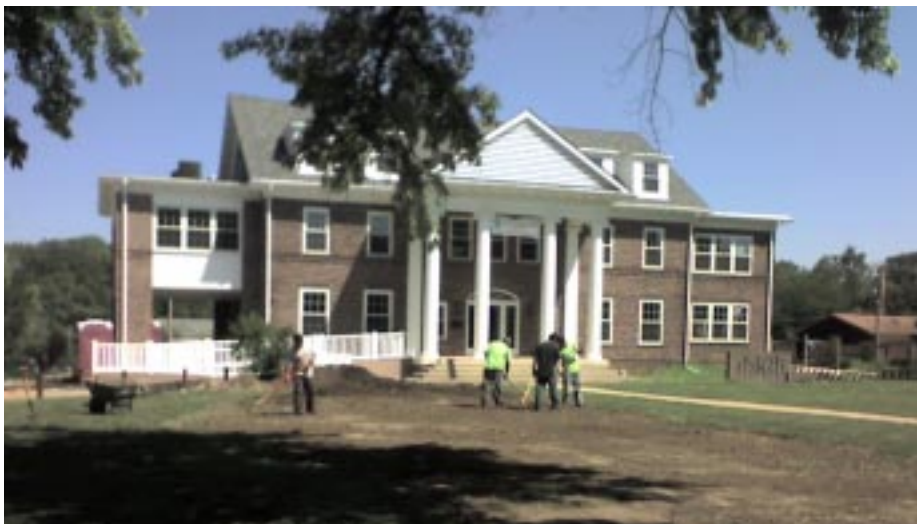
Landscaping work around the house, front yard taken from the street, August 5, 2006.
