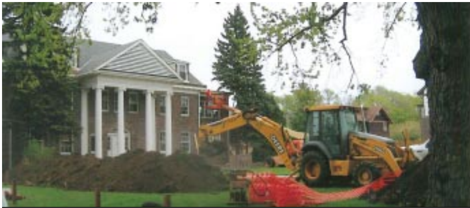
Putting in the fire service line for the sprinkler system and fixing the soffits
